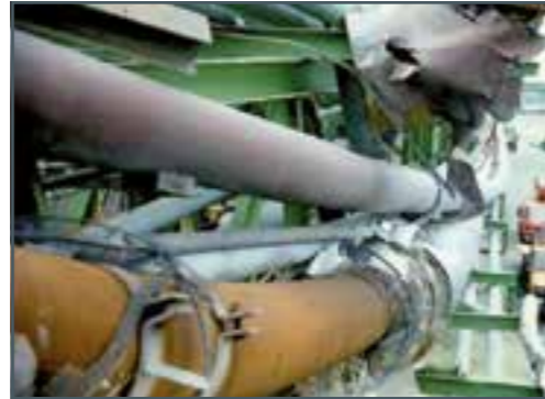
Damaged pipe and pipe brackets caused by a water hammer
