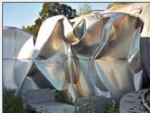
Collapsed tank as a result of water hammer
