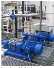
Pumps to circulate the oil
